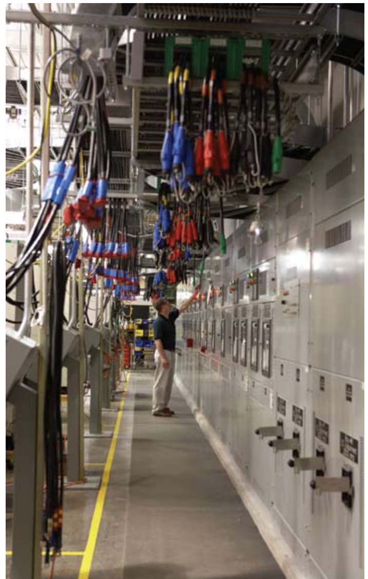
Eaton's Witness Test Centers allow you to see your large multi-module system tested before it is deployed.
