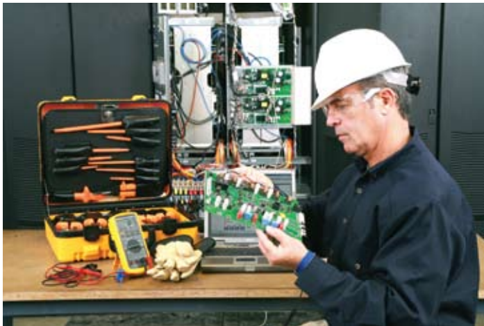
Proper preventive maintenance reduces the risk of UPS failure through thorough inspection, cleaning, testing and calibrating the various electronic and mechanical components of a UPS.
